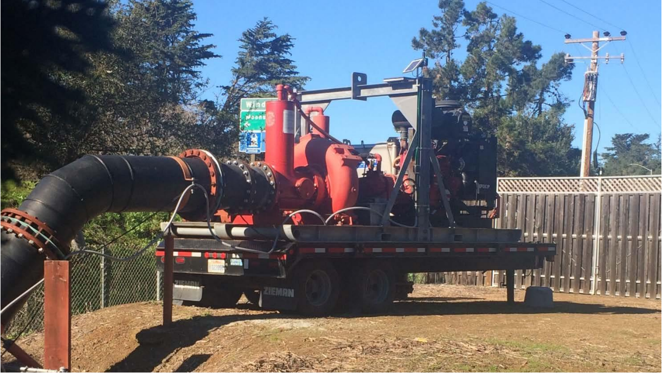
Flood Pump on Main Street - West Village
