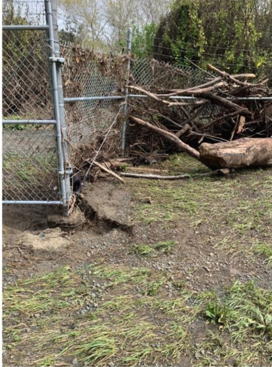
Figure 9 Lift station B log jam
