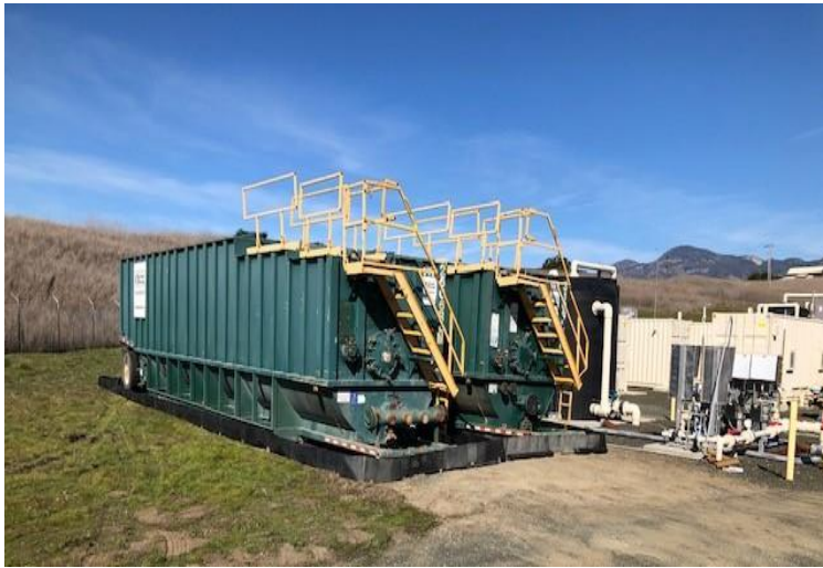
Figure 5 Newly installed brine storage tanks at the SWF
