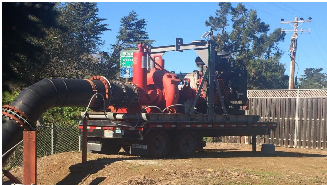
Flood Pump on Main Street - West Village
