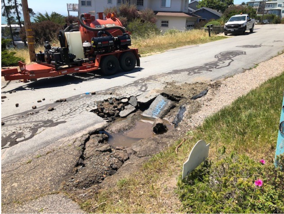
Figure 3 Condition of Emmons St valve failure upon arrival.
