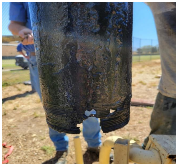
Figure A - SR4 well casing with corrosion at 81' below surface. This failure allowed silt to enter the suction pipe, contributing to failure of the pump impellers and motor and degraded water quality.
