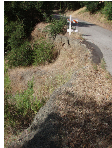
Erosion at Santa Rosa Creek Road
