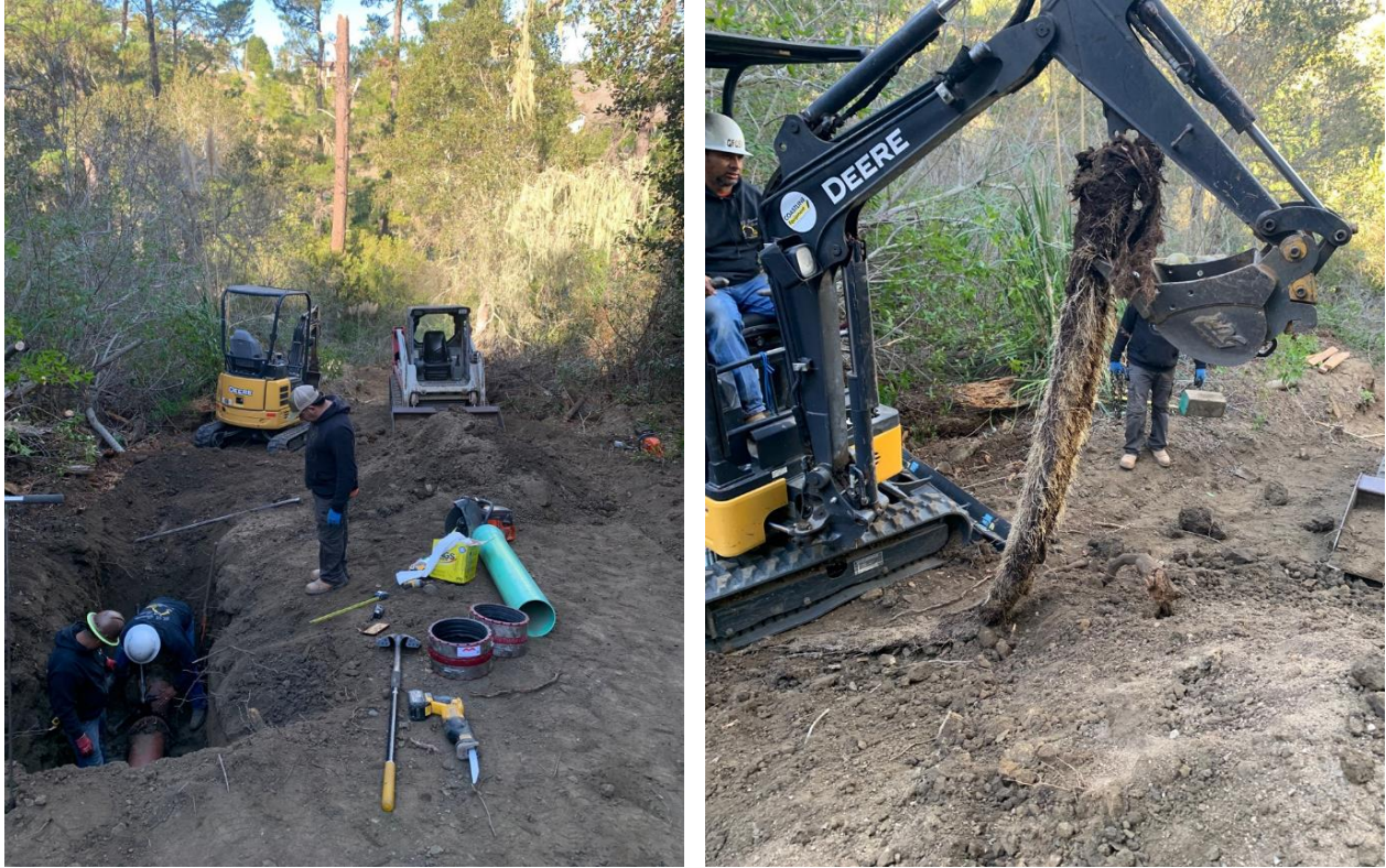
Figure B - Left: Excavation of the root intrusion near point of sanitary sewer overflow; Right: root intrusion removed from collection system
