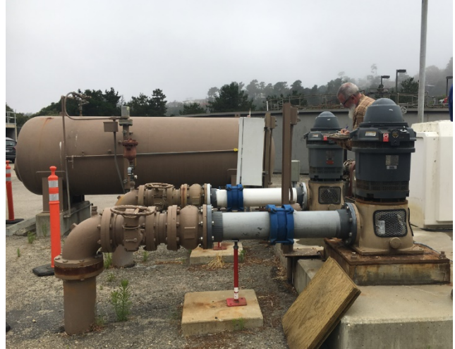
Figure 14: Effluent pump station
