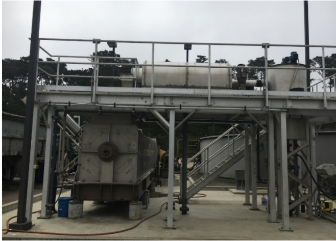
Figure 10: Sludge thickener and screw press
