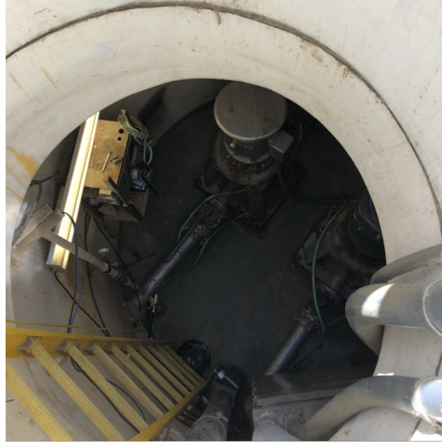
Figure 16: Lift station B4
