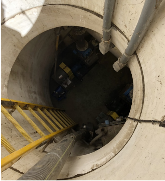
Figure 15: Lift station B1
