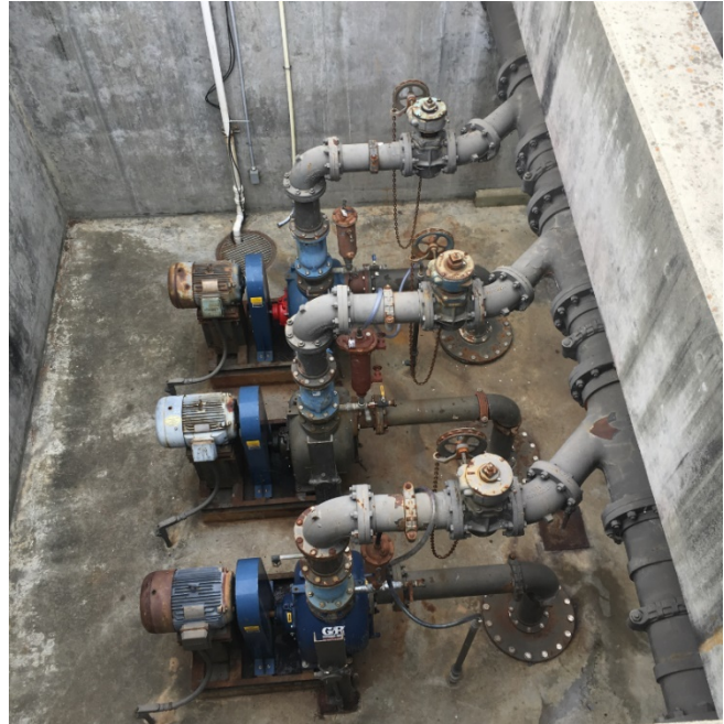
Figure 4: Influent pump station
