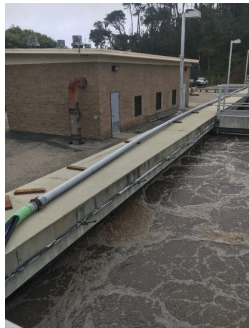
Figure 5: Aeration basin and blower building
