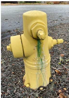
Figure D - Faulty Fire Hydrant (Subsequently Replaced)
