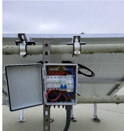
Figure C - Pineknolls Solar Panels with Battery Storage
