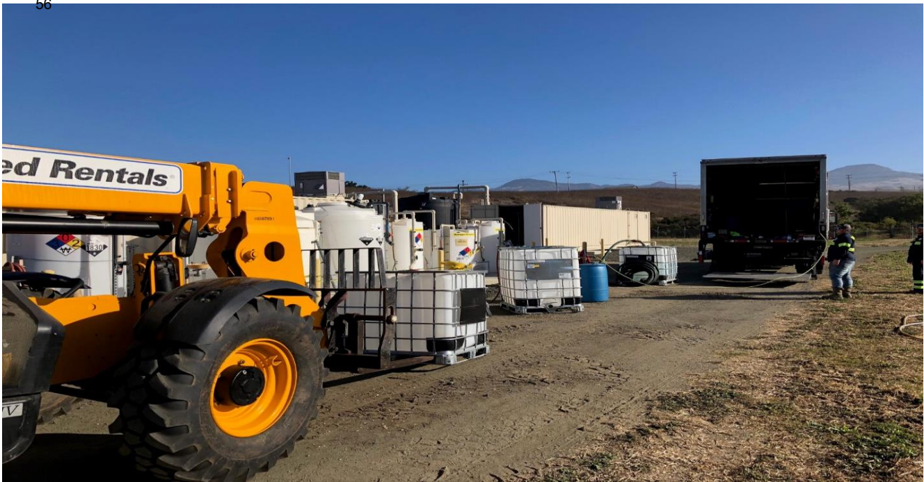
Photo of Recent Work by Chemical Supplier Brenntag in Replacing the Sodium Hypochlorite tank, which had a bad fitting.
