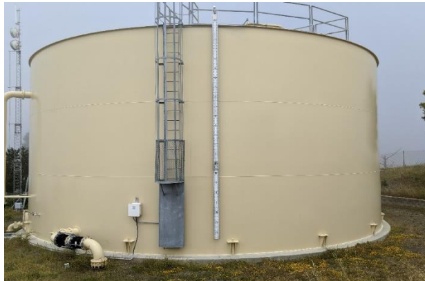
Figure 4 Fiscalini 120,000 Gallon Storage Tank
