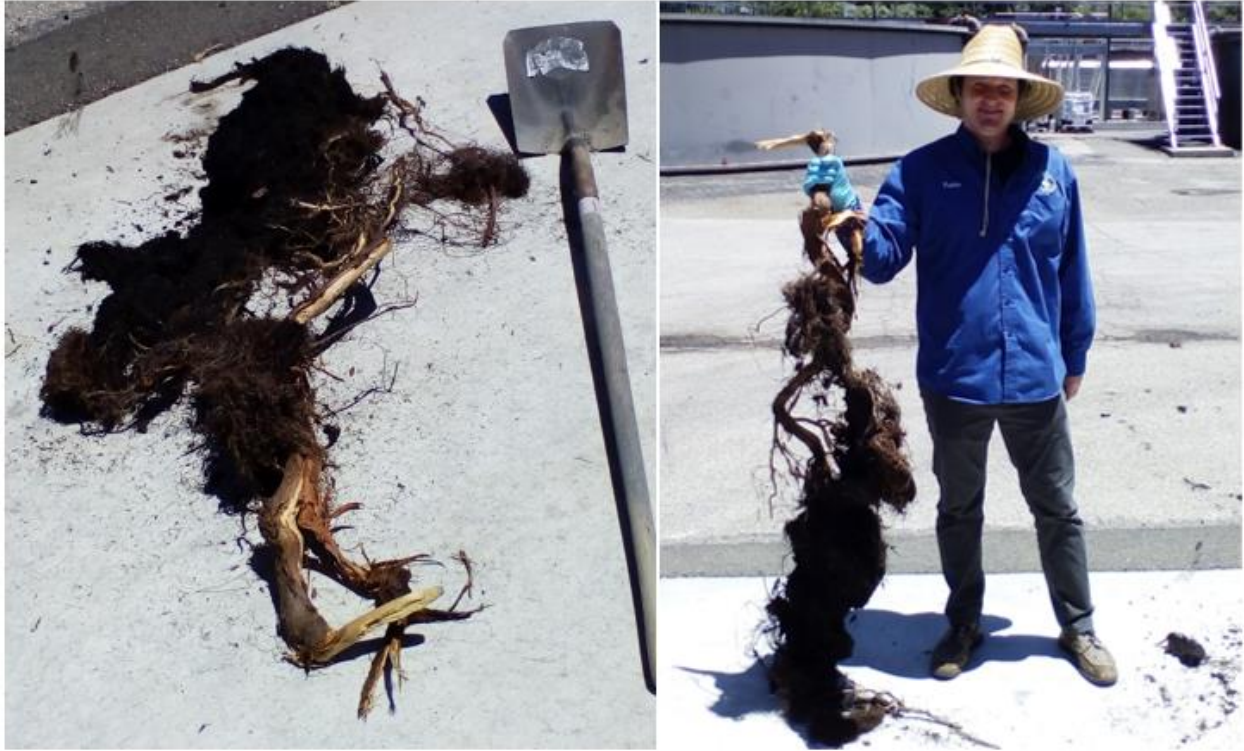
Figure 3 Root excavated from collection system lateral. Quite the catch.
