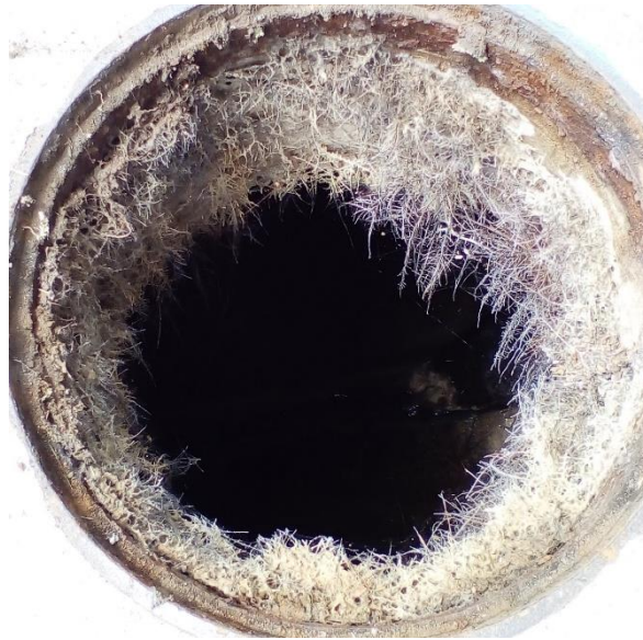
Figure 4 This is a manhole that had been covered up for many years.
