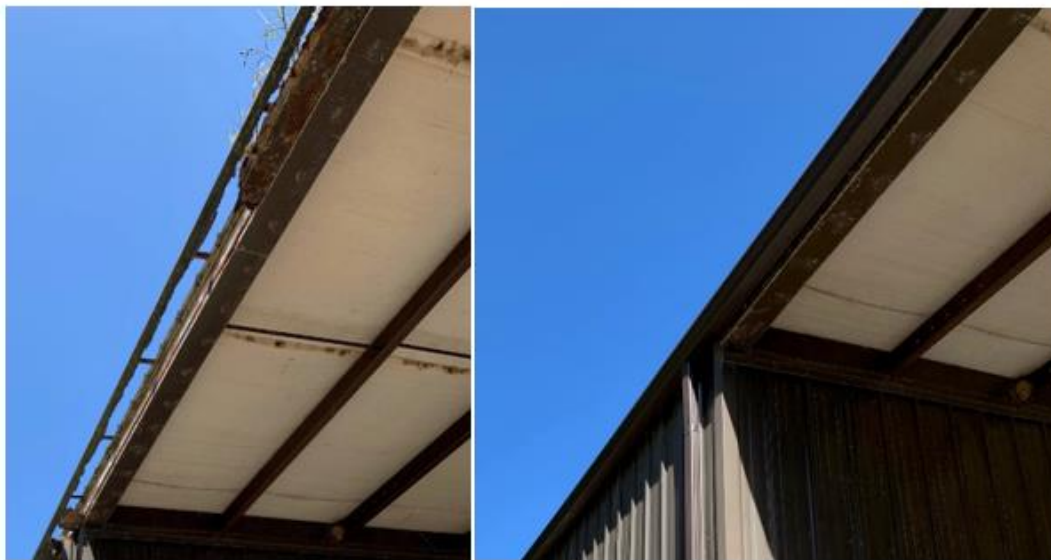
Figure 2 Before (left) and After (right) Rain Gutter Replacement. The vendor also replaced the down drains.
