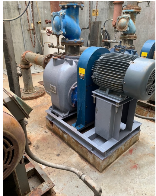
Figure A - Influent Pump #2
