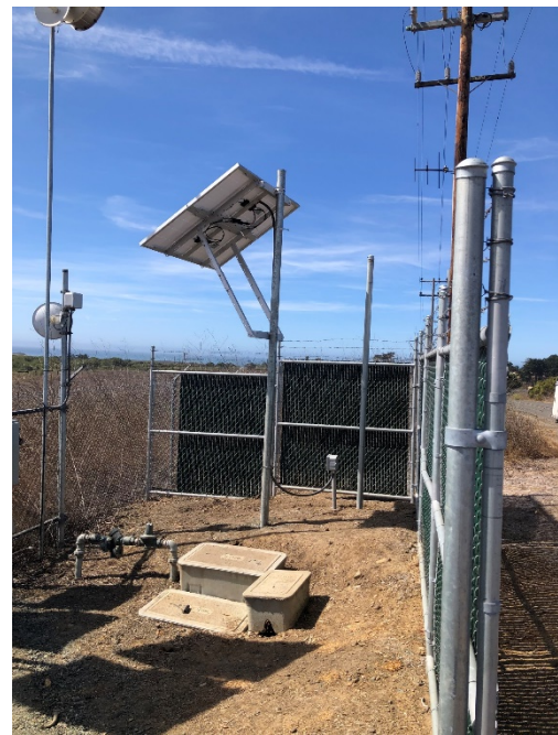
Figure E - Solar-powered Relay Station
