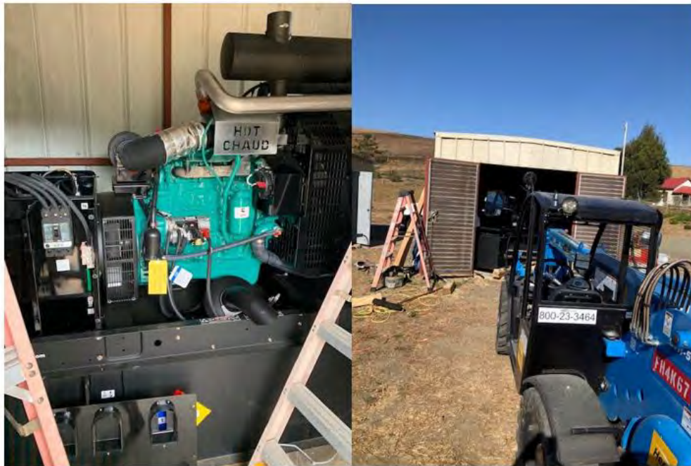
Figure 1 New Generator (left); Installation (right)
