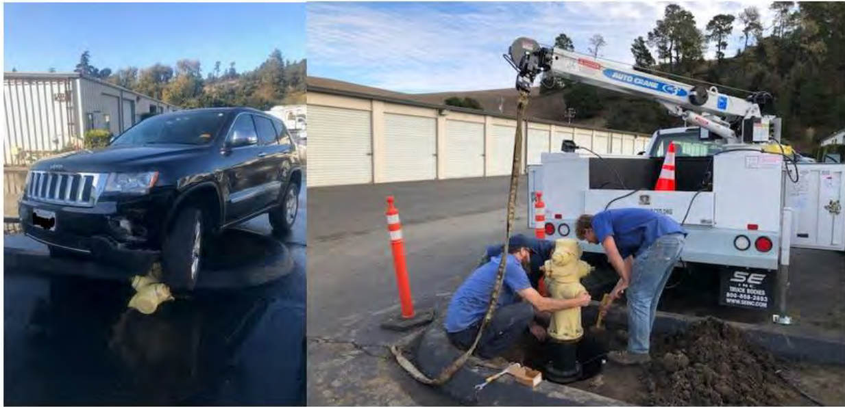
Figure 2 Fire hydrant incident (left); Hydrant repair (right) (Operators Andy Lyman and Adam Steventon pictured)
