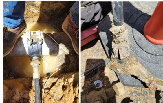
Figure C - Corroded saddle on Banbury Rd before (right) and after replacement (left)
