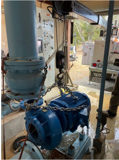
Figure F - Fire flow pump installation at the Leimert Booster Station
