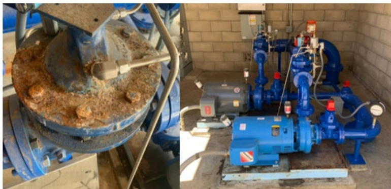
Figure D - Pipe condition before (left) and after (right) maintenance
