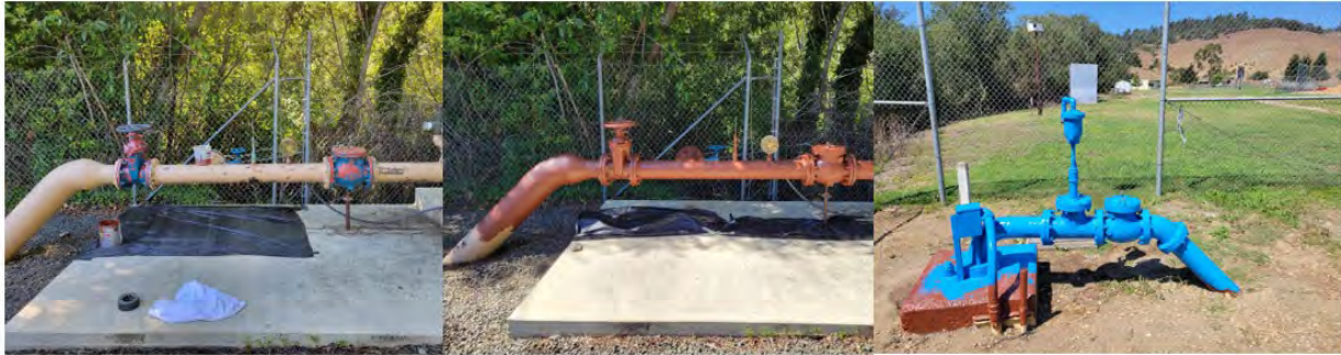
Figure E - Before exterior coating application (left), metal primer application (center), and finished two-part epoxy coating (right)
