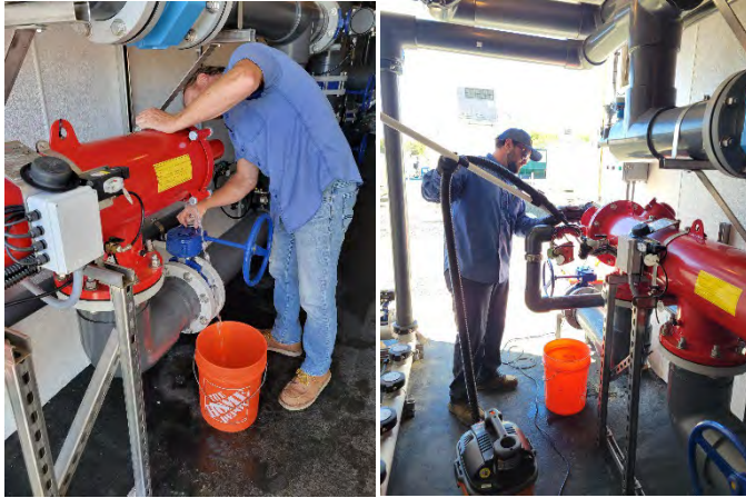
Figure G - Water Systems Superintendent Jim Green (left) and Operator Cody Meeks (right) perform maintenance on the strainer filter
