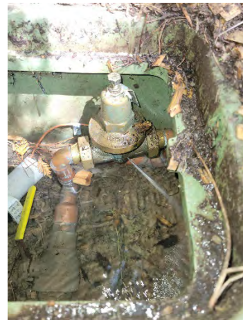
Figure D - Leaking Pressure Regulator at Cambria Pines Lodge
