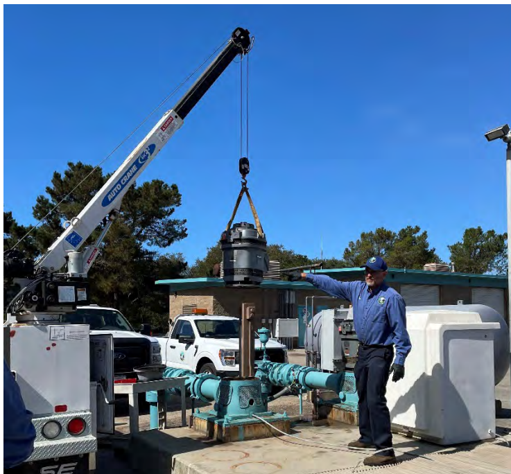
Figure A - Effluent Pump #2
