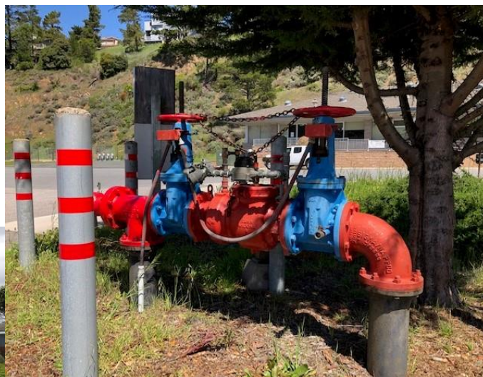
Figure 3 CCSD-owned backflow assembly
