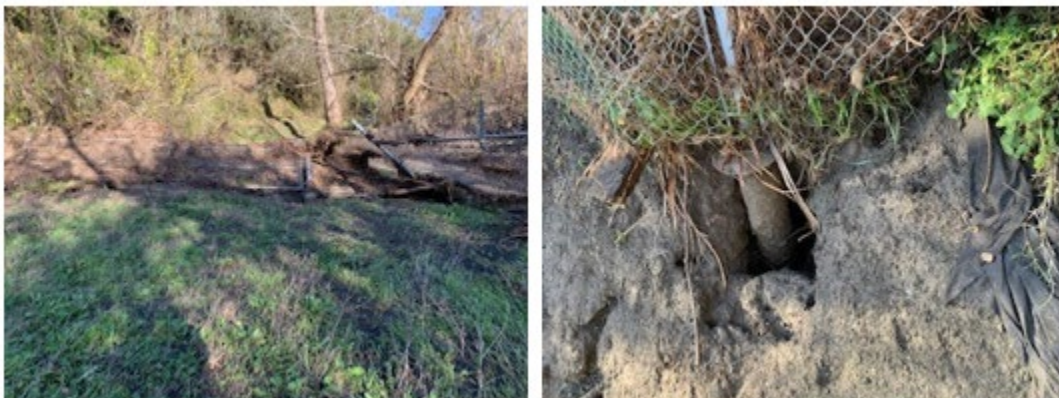
Figure E Storm damage at Lift Station B
