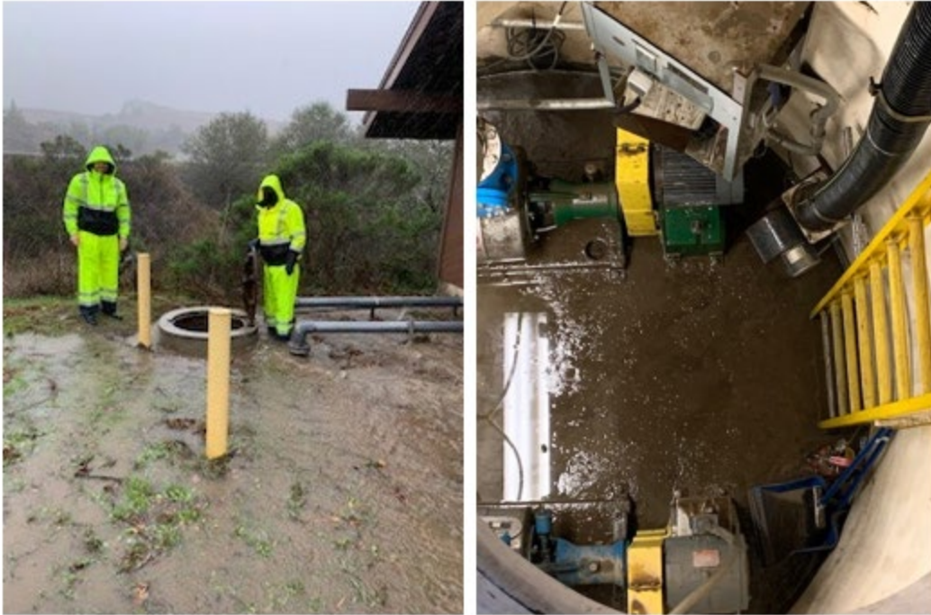
Figure D Staff at Lift Station B3 (left); muddy water at the bottom of lift station B1 (right)
