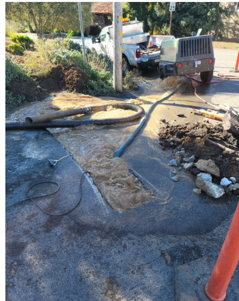
Figure F Dead end cap failure at Canterbury
