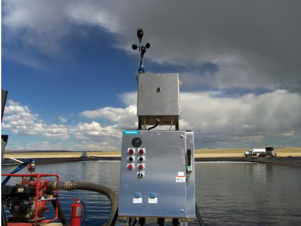
Figure 2-11 Weather Station Control Panel
