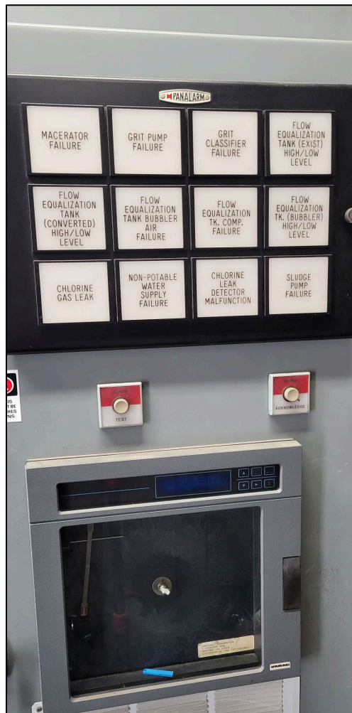
Figure 8: 1980's Era Analog Control Panel
