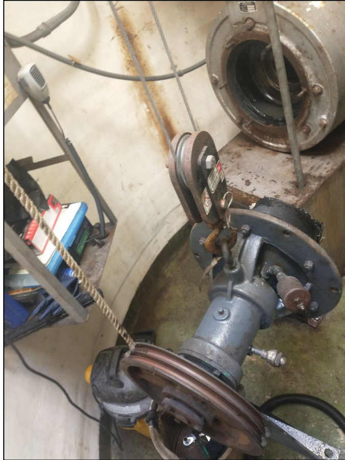
Figure 11: Rotary Assembly From Lift Station A
