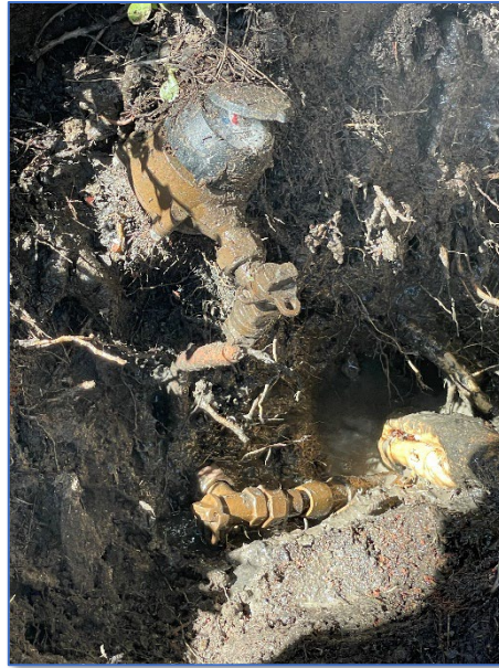
Figure 9: Burton Drive root damage to water service line
