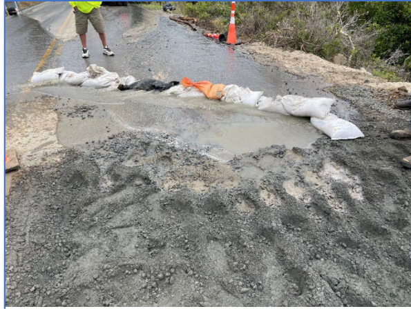
Figure 5: Pineknolls Drive water leak
