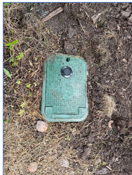
Figure 14: CCSD Water Meter box (Closed)
