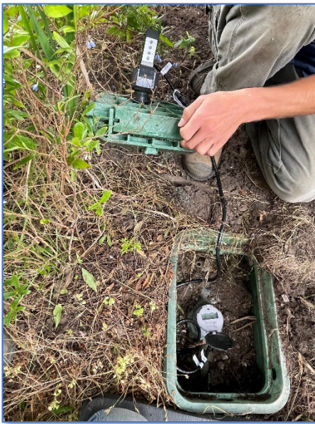
Figure 13: CCSD Water Meter box (Open)
