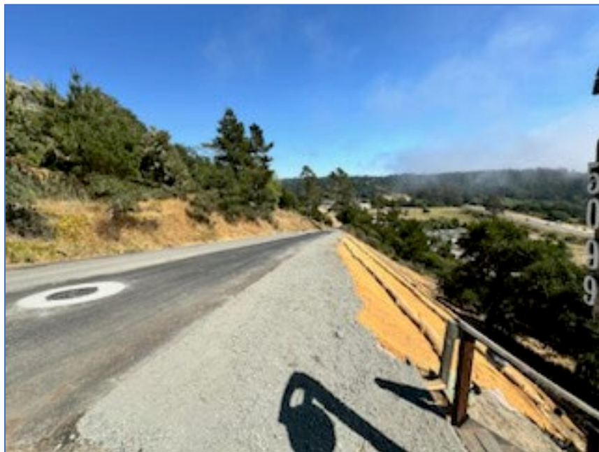
Figure 3: Pineknolls Drive and hillside repair
