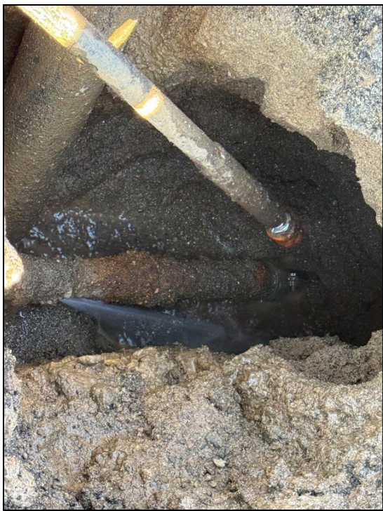
Figure 4: Rusted and leaking pipes on Moonstone
