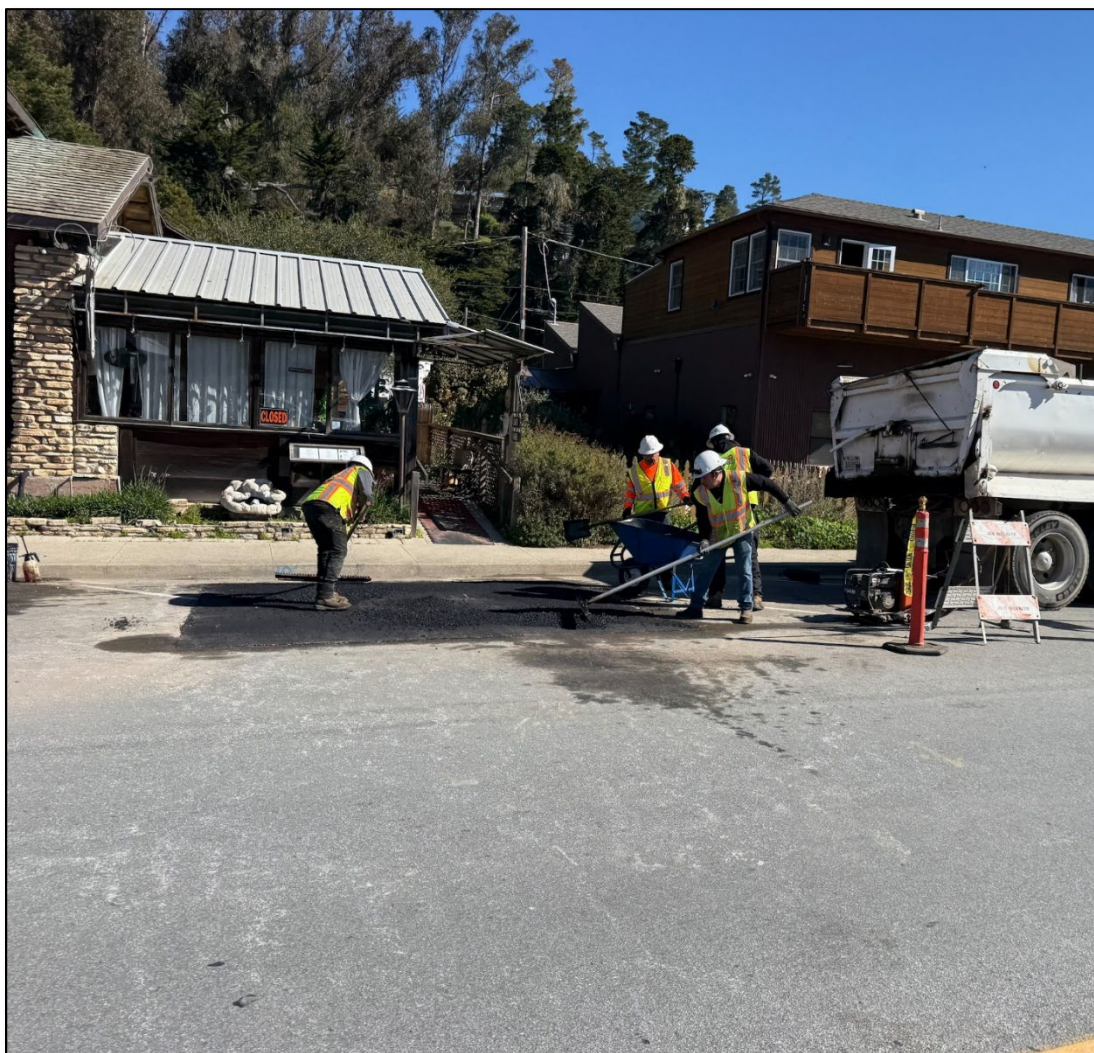
Figure 8: Patching on Main Street
