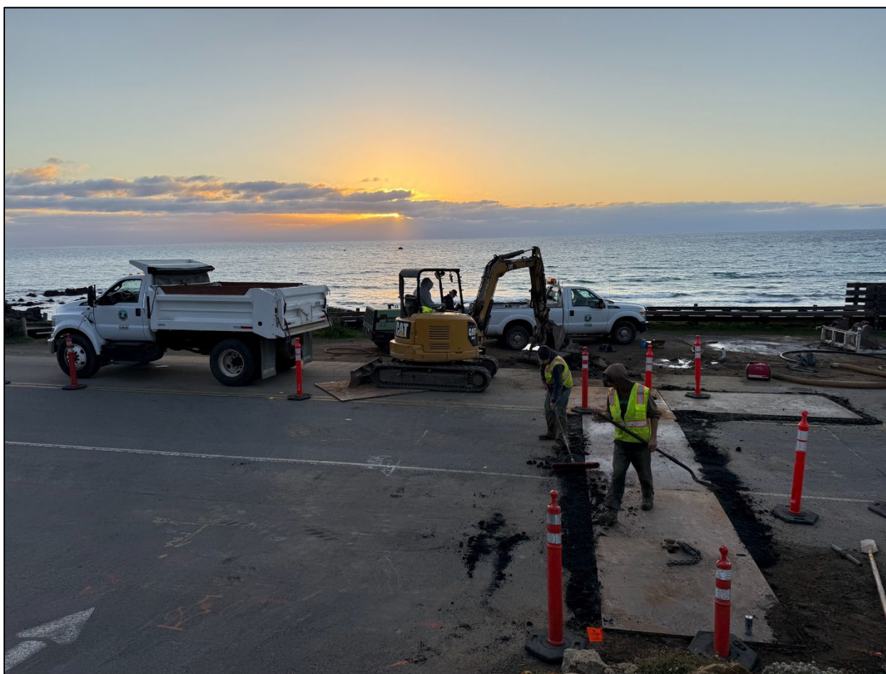
Figure 7: End of the day clean up to keep the Moonstone Drive in service
