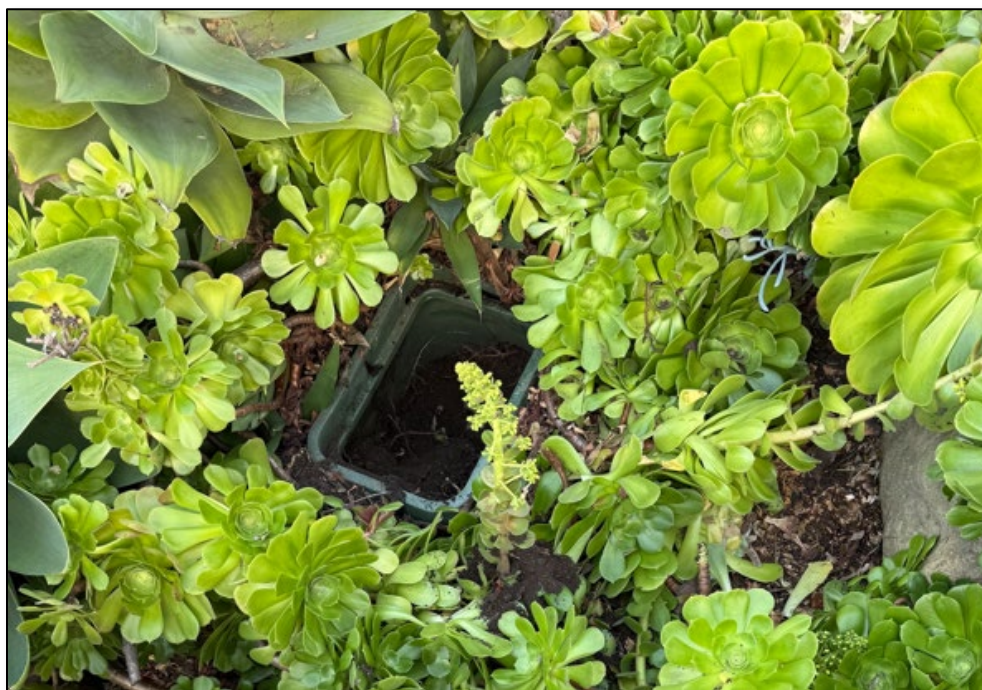
Figure 19: Meter box in need of clearing
