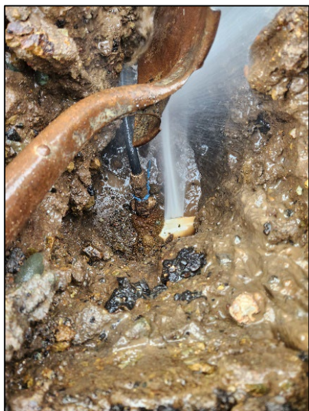
Figure 9: Cracked water main
