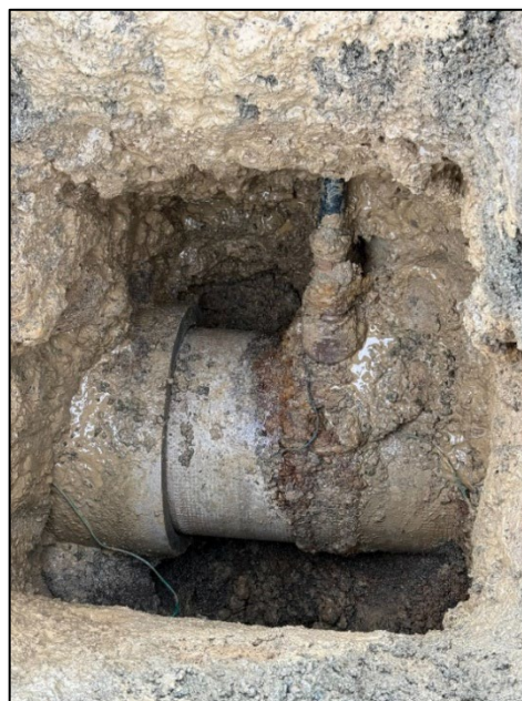
Figure 6: Rusted saddle connection
